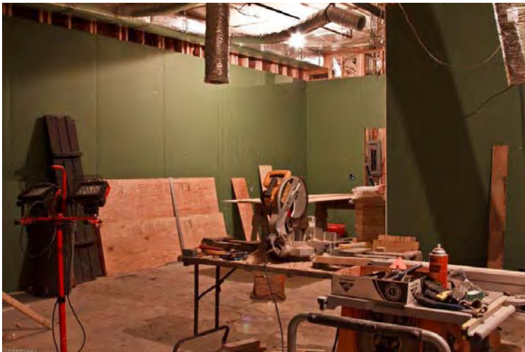
Work going on in the old Dorris/Cheek Drugstore, which will become the new “Research Library”
