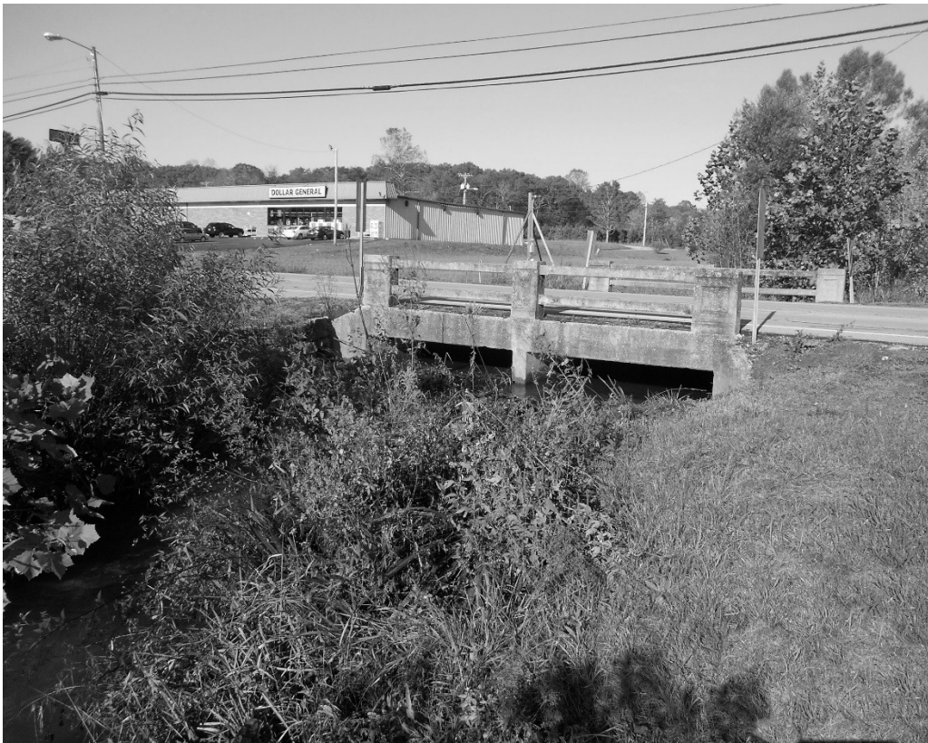
Colyar Stree Bridge across Happy Bottom creek in Tracy City.” This view is from The Lunch Box looking toward the Dollar General store.
